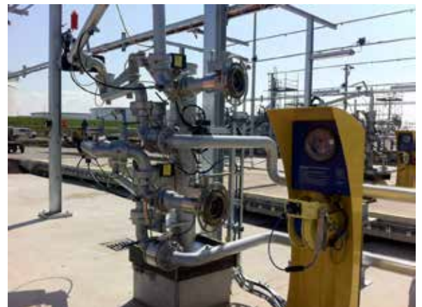
LPG loading facility
