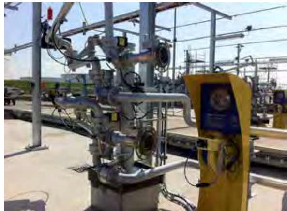
LPG loading facility
